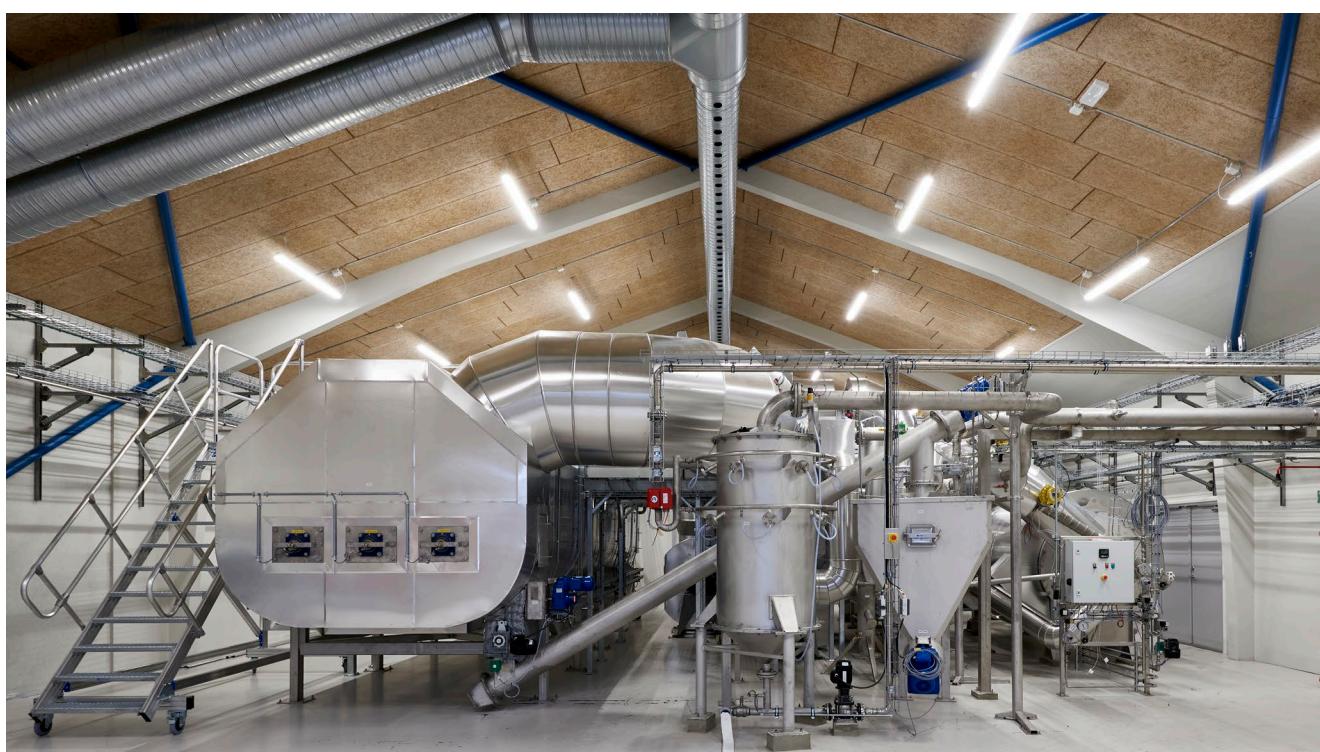
Figure 33: Picture of AquaGreen HECLA plant for steam drying and pyrolysis of sewage sludge in Fårevejle, Denmark. Picture is taken during construction. Today the plant is in full operation. © AquaGreen
